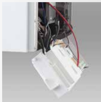
Opening of the panel board
