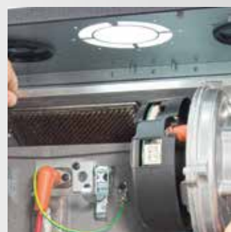
Opening of the complete combustion system
